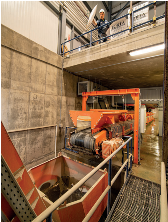
The WCS allows the batch plant operator to manually add specialty components, such as structural fiber or pigments, into the skip bucket for delivery to the mixer.
