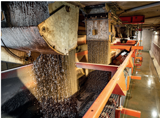
A weigh belt below the aggregate bunkers, with dual batch gates, for coarse fine batching, accurately weighs up the aggregate batch. Additionally, the geothermal temperature of the below grade bunkers benefits both winter and summer concrete production.
