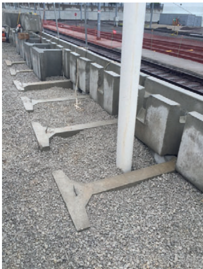
MagnumStone's extender system enabled the installer to work around existing utility poles, saving time and money.
