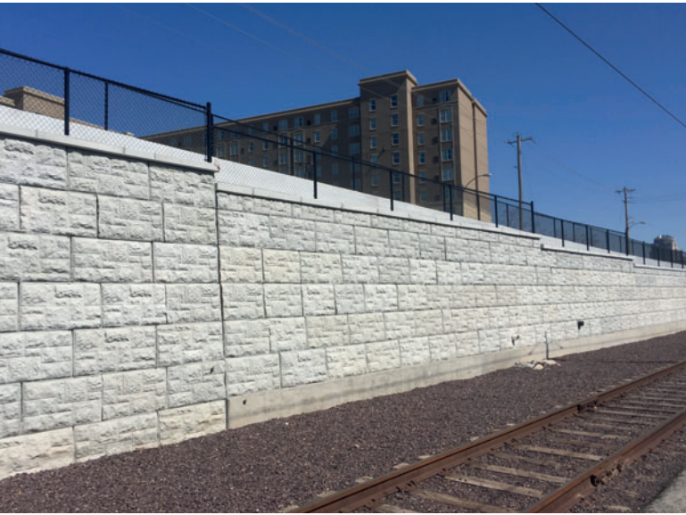
With a St. Louis city street above and a working railyard below, installers had a tight footprint in which to erect the retaining wall.
