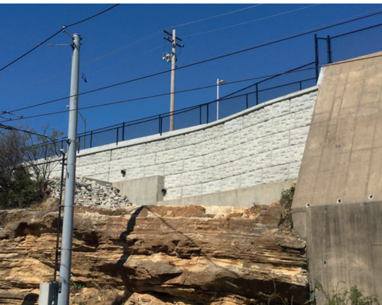
The flexibility provided by the MagnumStone system enabled the new retaining wall to be installed around existing utilities and join up with remnants of the factory foundation.
