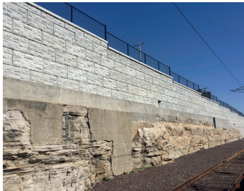
Blending the modern retaining wall with the remaining historic structure gives the MetroLink site a truly unique design.
